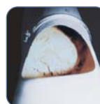
Blocked up pipes which fumigation gases cannot penetrate.
